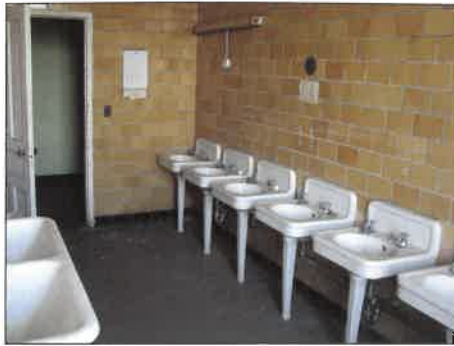
A portion of the second floor toilet and shower facility. Despite the building's age, it retains many of its original features and fittings, including this row of sinks. COURTESY NYSOPRHP, DOUGLAS W. DeCROIX PHOTO
